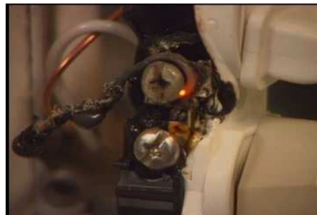
Fig. 4, Demonstration of glowing wire at a poor / loose binding screw connection, 14Amps, 14 AWG solid wire.
